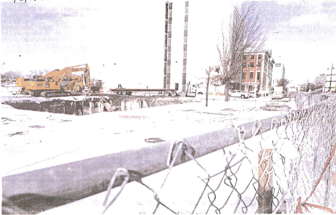
The site of the former Nelson House Hotel Annex on Wednesday on Market Street in the City of Poughkeepsie. Workers will begin filling the basement with gravel next week. They will then spread seed, topsoil and straw mulch. DARRYL BAUTISTA/POUGHKEEPSIE JOURNAL
